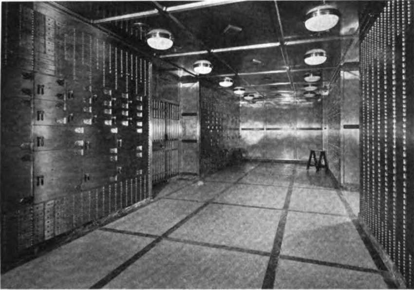
A view of the interior of the safe deposit vault in the new building of the Pennsylvania Company for Insurances on Lives and Granting Annuities, Philadelphia, Pa. The vault was built by the Mosler Safe Co., Hamilton, Ohio.
