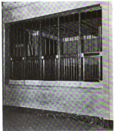
Detail of built-in grille, showing bronze work, Atlantic National Bank, Boston. By William H Jackson Company
