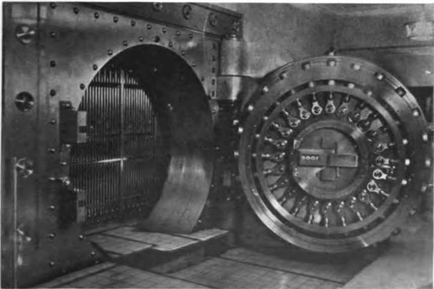
Entrance to the new vaults of the State Bank of Chicago. The vault door alone weighs more than 125,000 pounds. It was installed by the Mosler Safe Company, Hamilton, Ohio.
