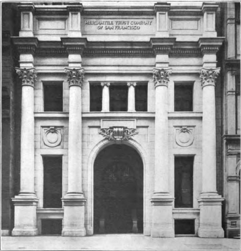
MERCANTILE TRUST COMPANY. Building damaged, but office still maintained therein.
