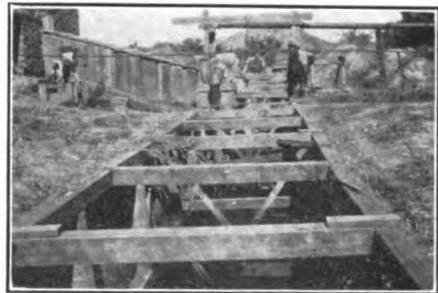
Section of Open Cut, 20 feet deep, 80 feet long, furnishing abundant water to irrigate 500 acres.
