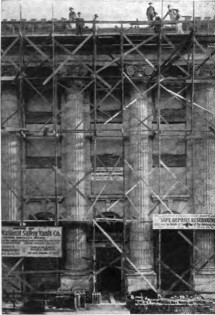
Building in course of construction for the National Safety Vault Co. of Denver, Colo.
