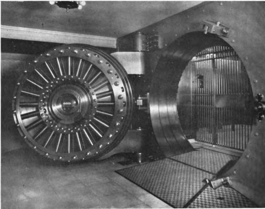
MAMMOTH VAULT DOOR OPEN, SHOWING BOLT WORK ESSEX COUNTY NATIONAL BANK, NEWARK, N. J.
