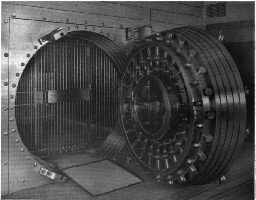
ANOTHER VIEW OF THE MAIN DOOR TO THE VAULTS OF THE NEW YORK COUNTY NATIONAL BANK—DOOR IS HALF CLOSED
