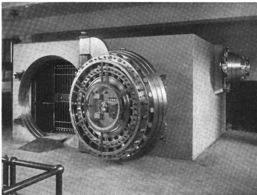
View of Armor Plate Vault made and installed by Bethlehem Steel Company for the E. P. Wilbur Trust Company, South Bethlehem, Pa.
